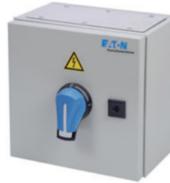
Door closed: operation with the external handle through the door.
